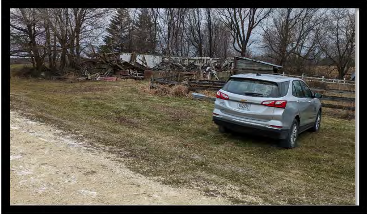
Collapsed barn proposed to be rebuilt for all-weather space and commercial kitchen southwest of dwelling. Wild Turkey Road is in the background behind the trees and the vehicle is parked in a proposed parking area.
