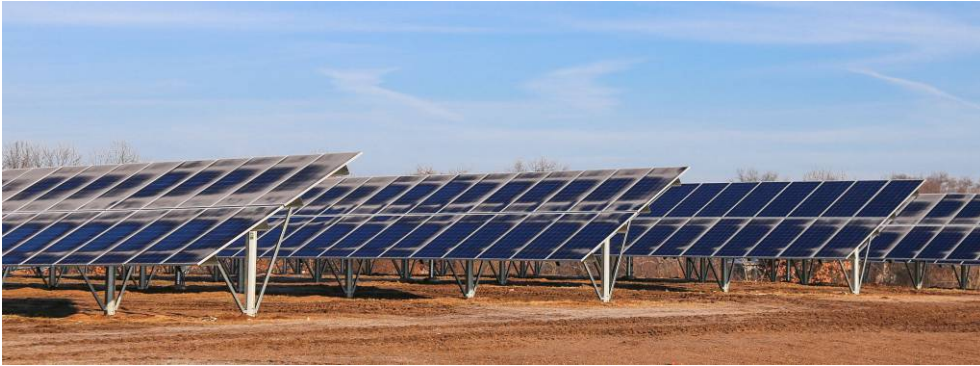
Typical Solar Arrays
