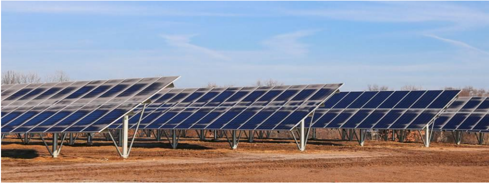
Typical Solar Arrays
