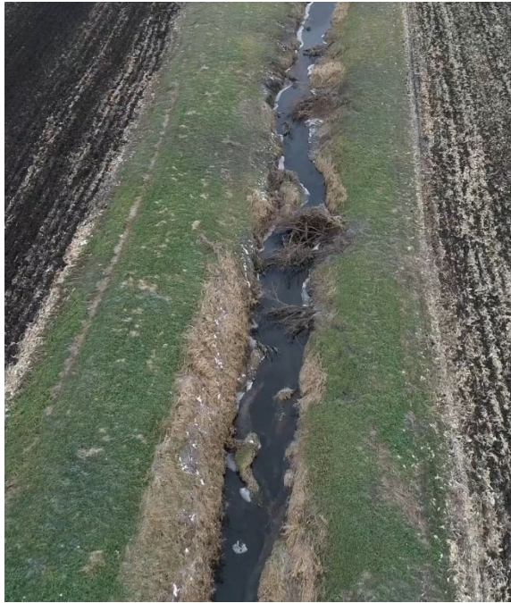
Vegetation Growth and Debris
