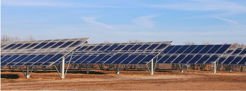
Typical Solar Arrays
