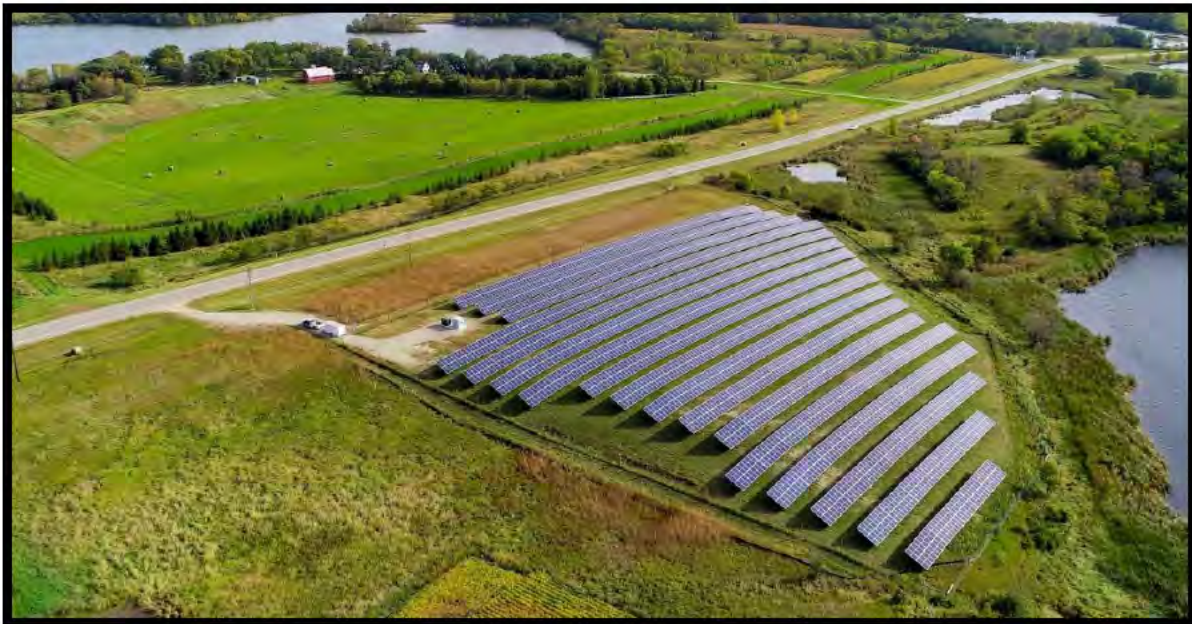
1MW CSG in Pope County
